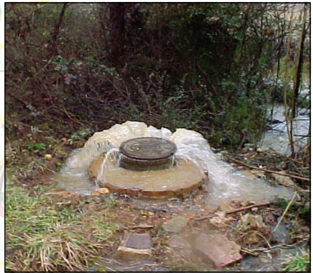
This is an actual sanitary sewer overflow caused by an oil and grease blockage.
